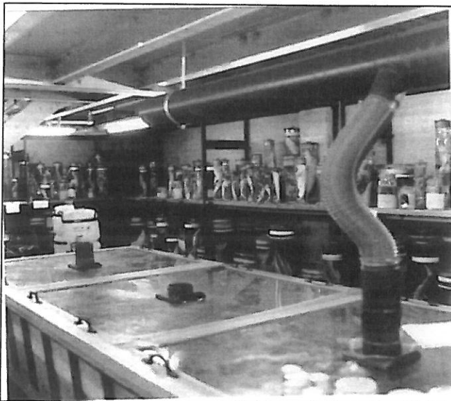
Fig. 3. A new spirit store room with open racking and vented tanks (photo from O. Crimmen).
