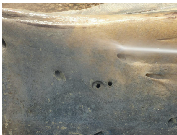
Figure 3. Cleaning tests with pressurized water designed to remove the black dirt under the paint. Image: © MCNB / ICP.
